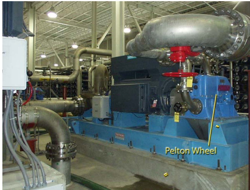
Figure 3 - Tampa Bay Desalination Plant Pelton Wheel Energy Recovery System
